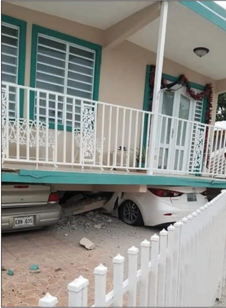
Photo 1. The series of daily earthquakes that struck Puerto Rico in late 2019 left buildings unstable and residents fearful for their safety. Photo courtesy of the Puerto Rico Department of Health.
