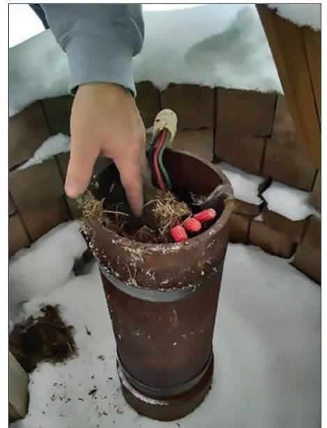
Broken well cap with mouse nesting material in Madison County, New York.
