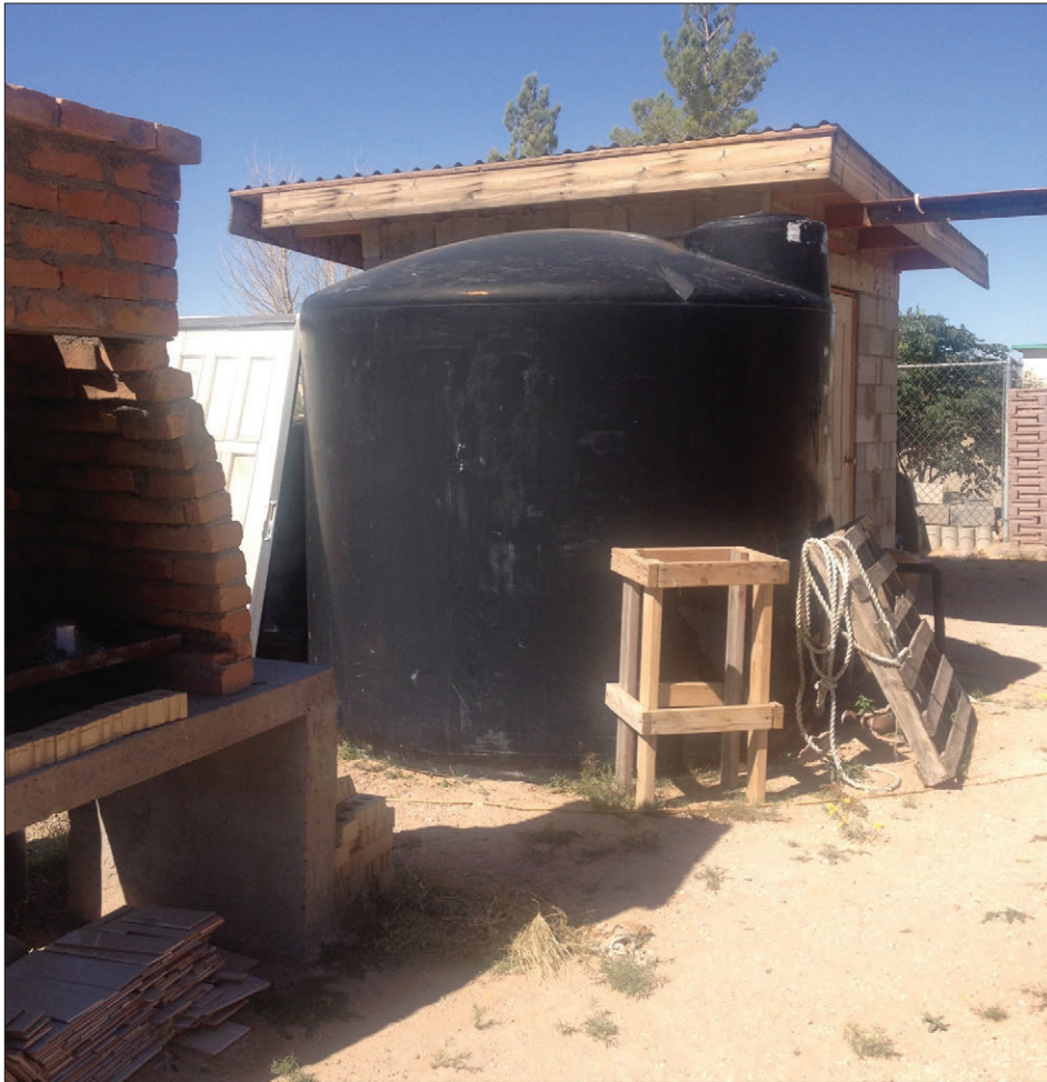
A typical hauled-water storage tank used by a colonia family in West Texas.
