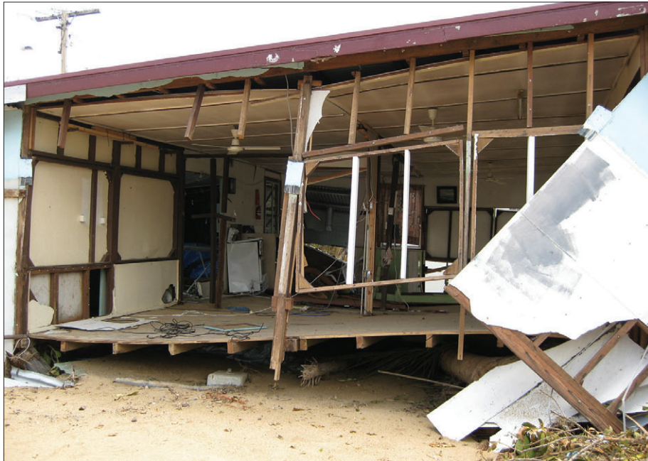
Impact of tidal surge—damage to external walls on the seaward side of a house.
